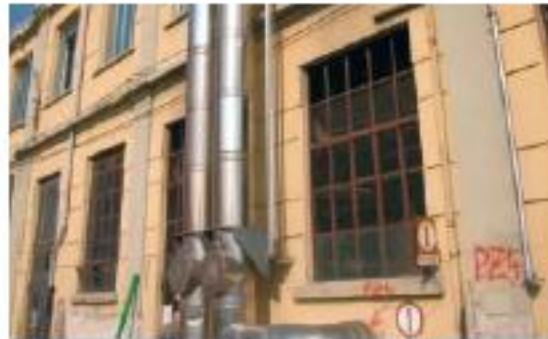
Aluminium pipes and office windows in the Pirelli building
