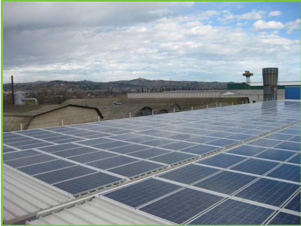
Installation on industrial rooftop
