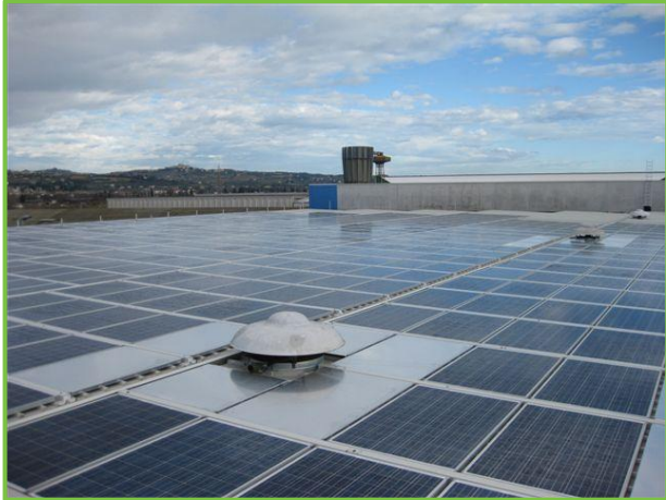
Installation on industrial rooftop
